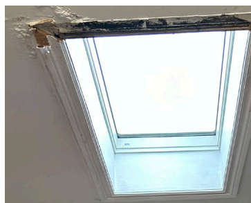
Skylight Water Damage
