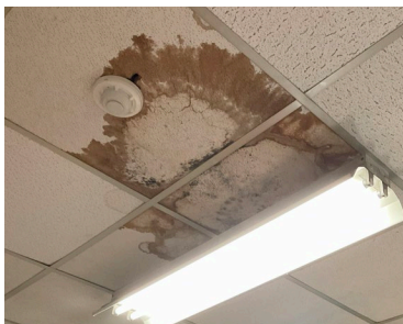
Bathroom Water Damage
