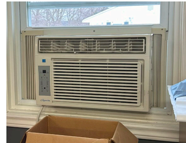
Window Air Conditioning Unit
