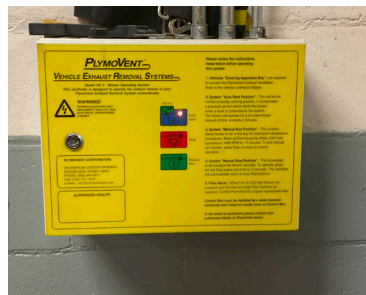
Vehicle Exhaust Ventilation System
